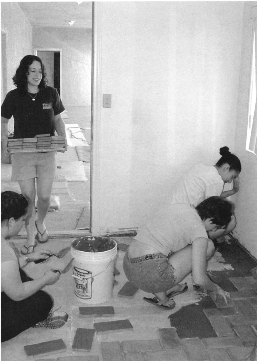
Left: There are so many details to take care of when you run a mission that ministers to homeless people. The Las Vegas team was able to pick up some of the easily overlooked but essential tasks like tiling this floor.
